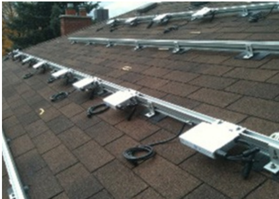
A Solar Electric Racking System
