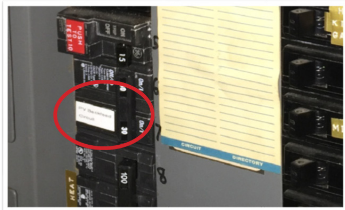
Photo 3: Working clearance not maintained: NEC 110.26
