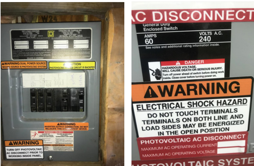
Photo 11: AC disconnect/load center manufacturer's label obscured: NEC 110.21
