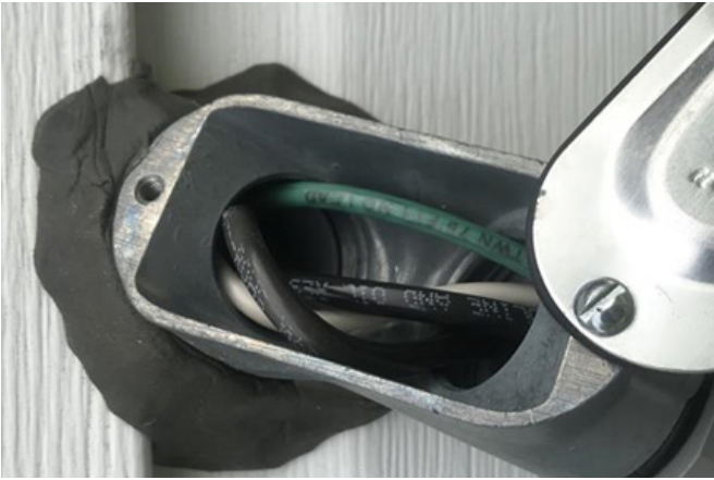
Photo 13: Two Hole conduit strap, with only one point of attachment, and no strain relief on conductors: NEC 110.3(B)
