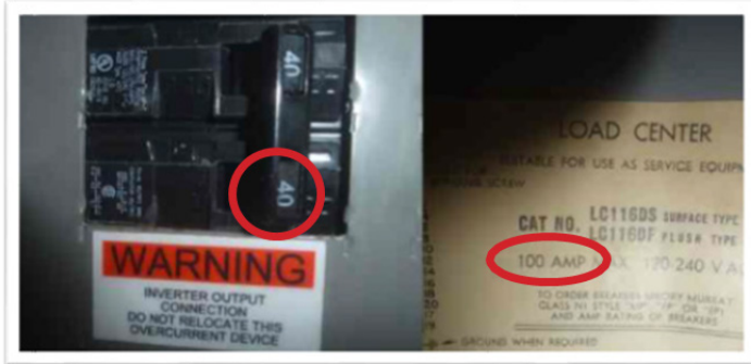
Photo 2: Backfed PV breaker not installed at opposite end of buss bar from main breaker: NEC 705.12(B)(3)(b)
