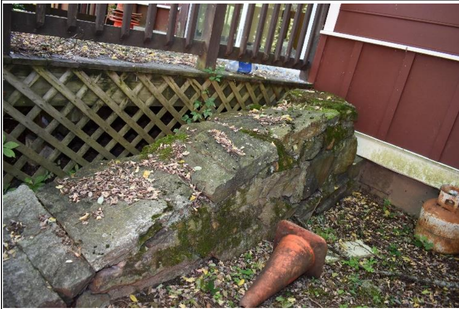
#17. The original barn had access to a second level, that has since been altered (Building E).
