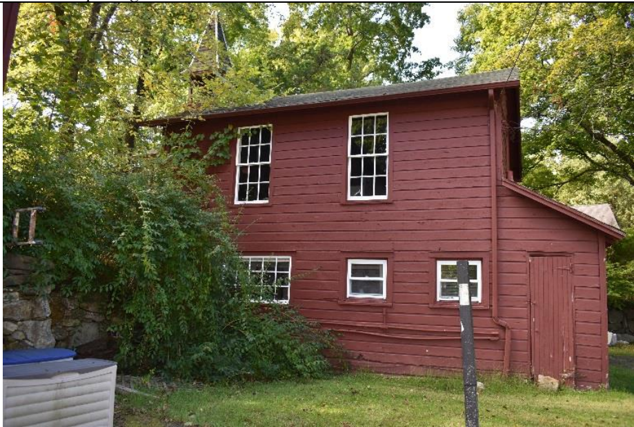
#31: Building H is constructed adjacent to a stone retaining wall. View to the west.
