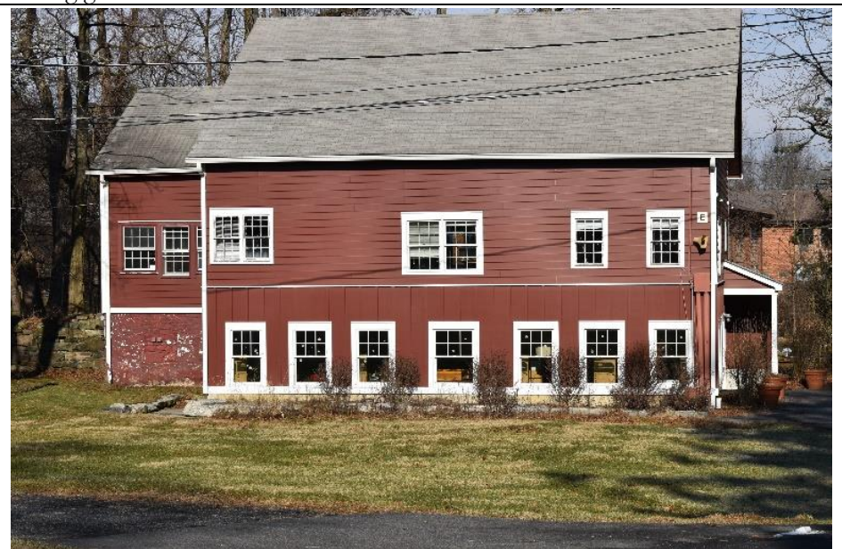
#20. Building E- The windows on the first level of the southern elevation are all modern vinyl replacements, and the second are irregular in placement.
