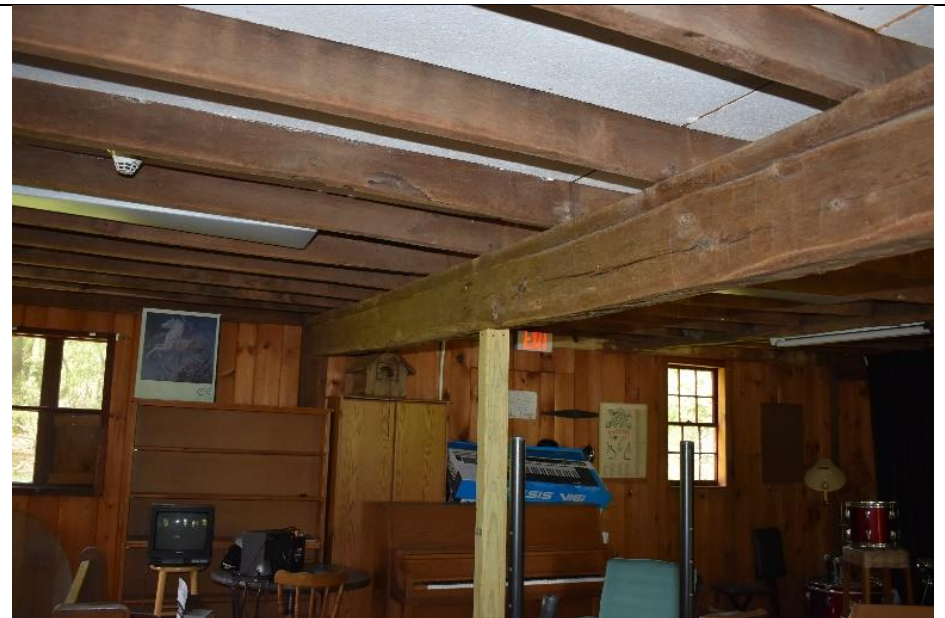
#40. The ceiling of Building I's interior is a mix of 20 th century lumber, timber beams and sheet rock.
