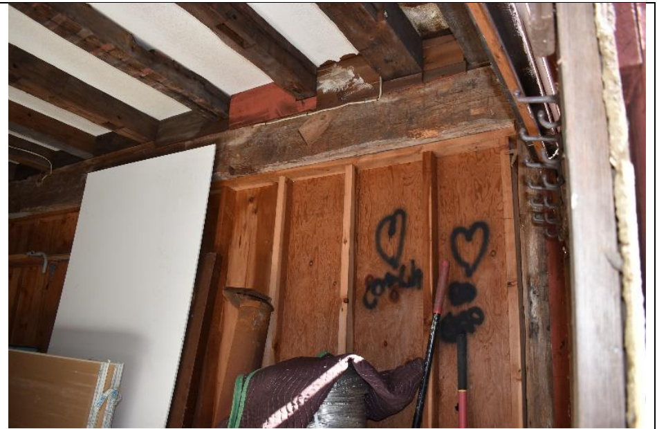
#30. The interior of Building G has been substantially altered into the 21 st century, with the addition of a framed interior wall.
