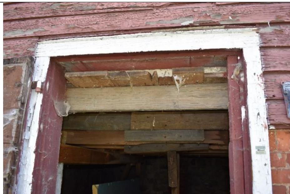
#2. The building materials in the basement are a mix of late 19 th century through 20 th century.
