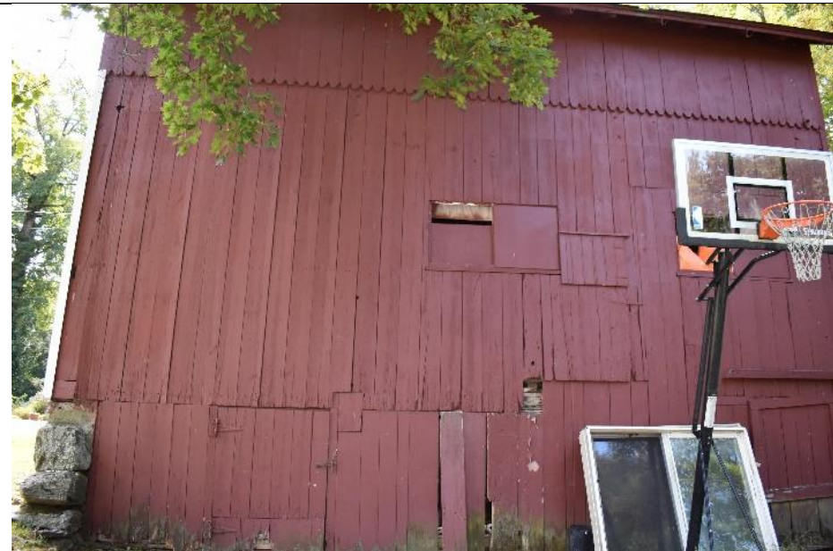
#23. Multiple openings and access points are visible on the northern elevation of Building G.
