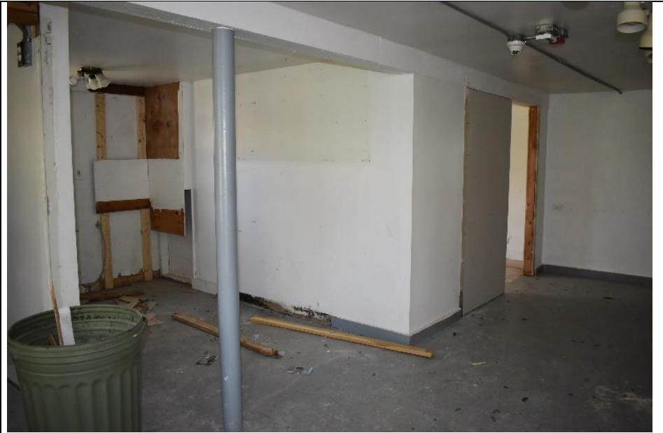
#34. The interior of the basement of Building H features a concrete floor, metal (steel) lally columns and other 20 th century materials.
