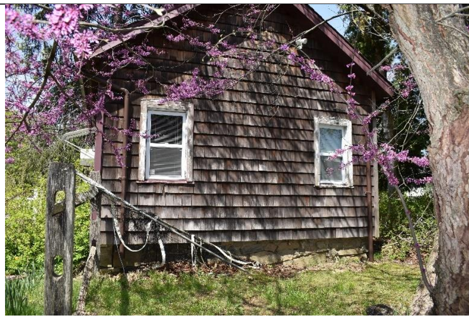
#4. The windows are modern vinyl replacements, and the siding style differs on the exterior.
