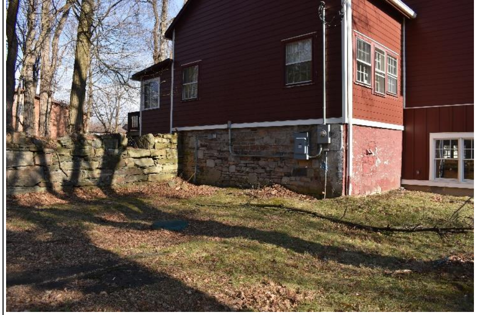
#16. Portions of the western foundation wall of Building E have been reconstructed using stone, possibly from the original barn.
