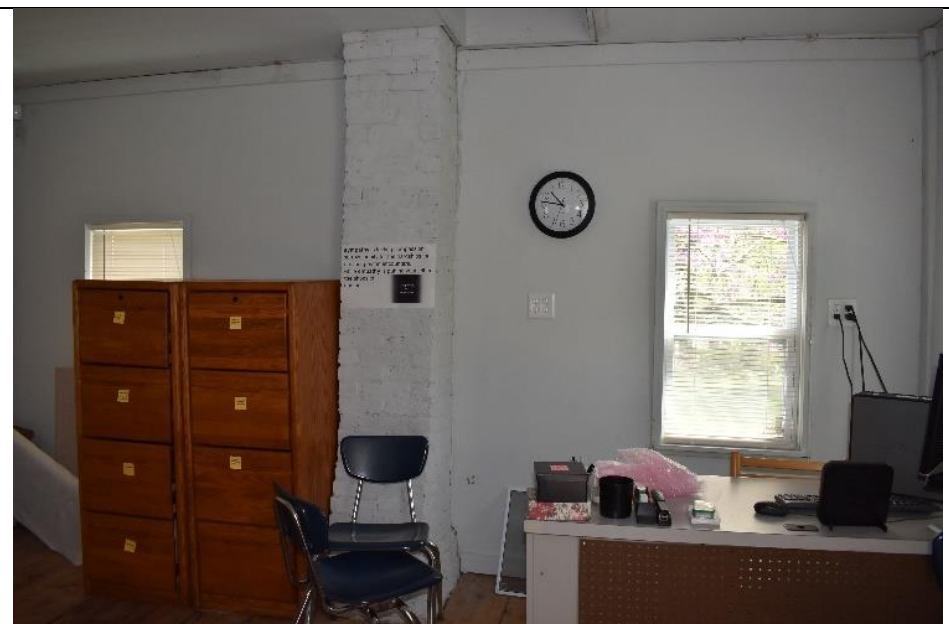
#3. The interior of the building has been substantially renovated, and includes modern materials.
