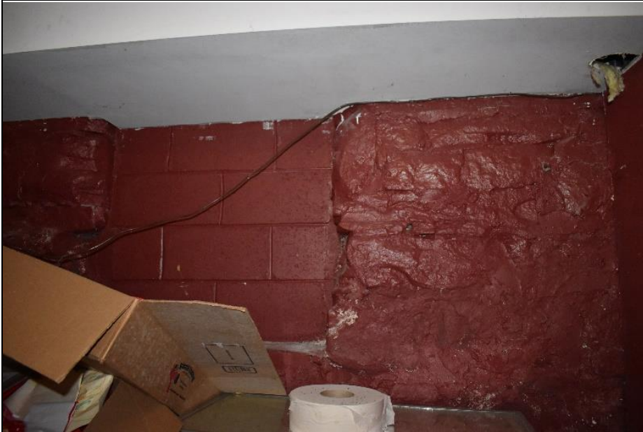
#11. The original stall openings, from the original use as a barn, have been closed up with cinderblock. View of north wall of Building E.
