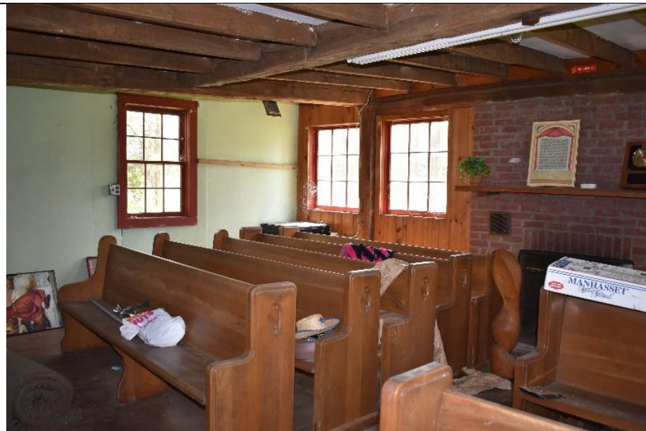
#39. The construction materials in Building I include timber beams, and 20 th century lumber, and 20 th century interior finishes.
