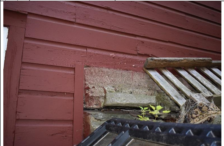
#36. Building H is partially fastened to a stone retaining wall on the southwestern corner.
