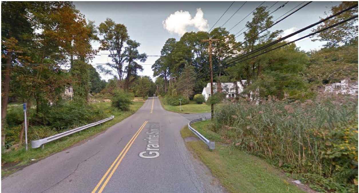
Photo 3. Granite Springs Rd with unnamed Class C watercourse flowing underneath through a culvert, between Gregory St and Broad St, facing east.
