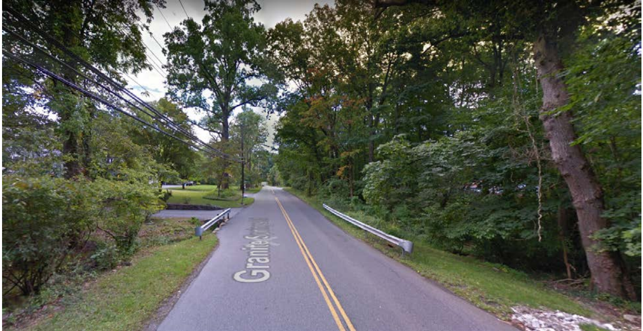
Photo 2. Granite Springs Rd with unnamed Class C watercourse flowing underneath through a culvert, between Barway Dr and Hedwig Dr, facing east.
