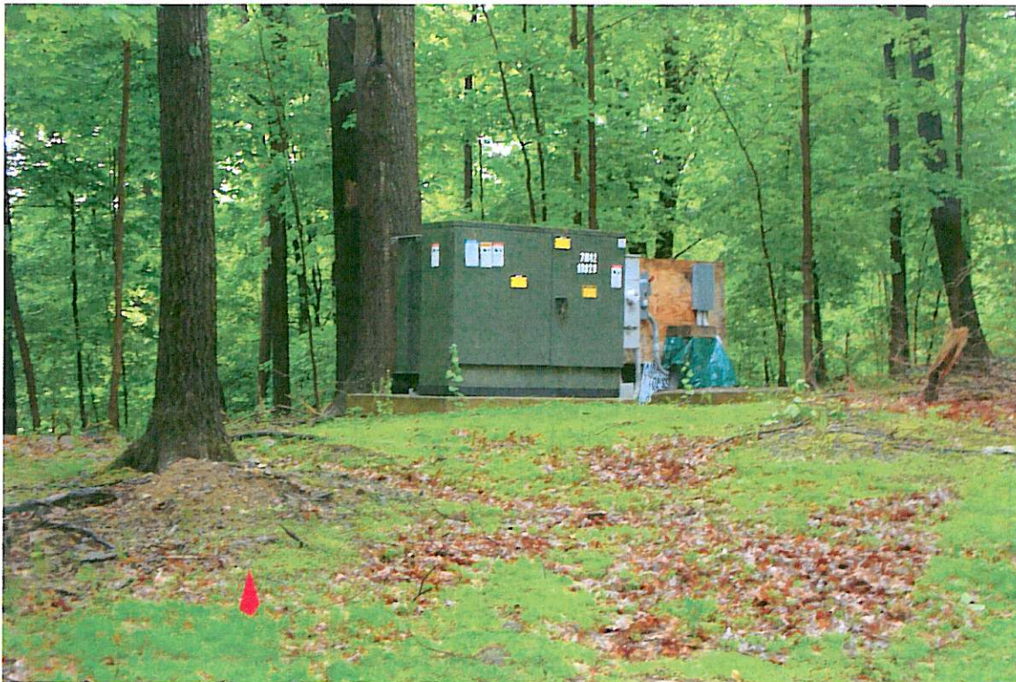
Photo No. 4 - View of on-site 240- to 480-volt transformer located upgradient of on-site ponds.
