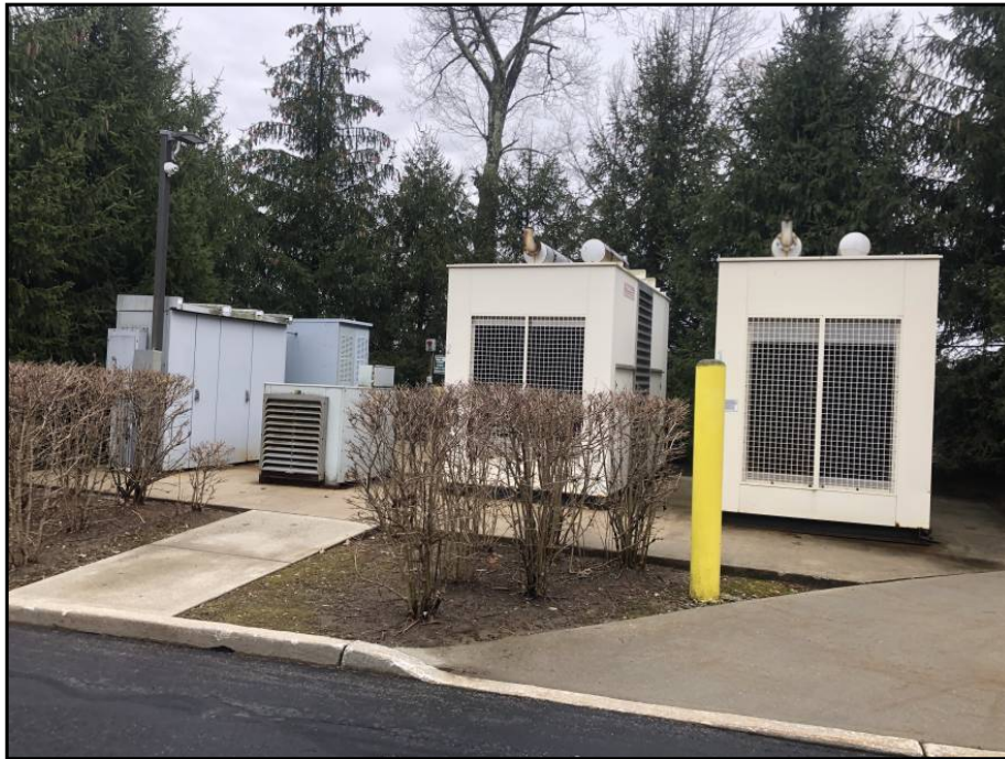
23 : Pad-mounted emergency generators
