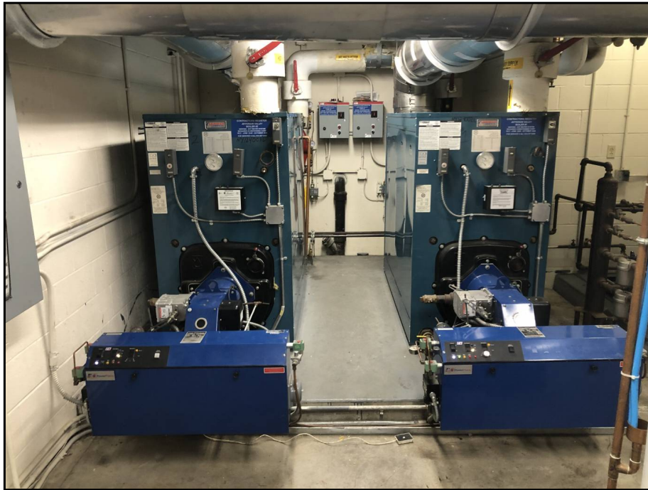
11 : Oil-fired boilers in boiler room of Building No. 2
