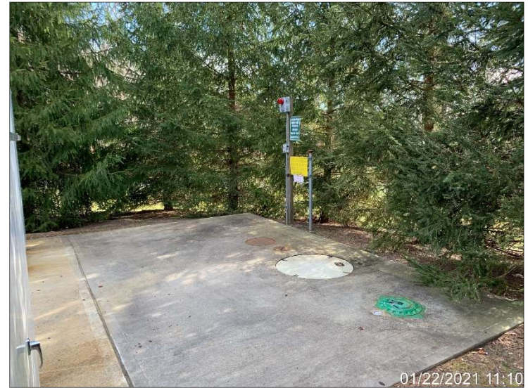
Photograph 30. 1,000-gallon No. 2 fuel oil UST (Tank No. 003) serving the two emergency generators, located behind the generators.
