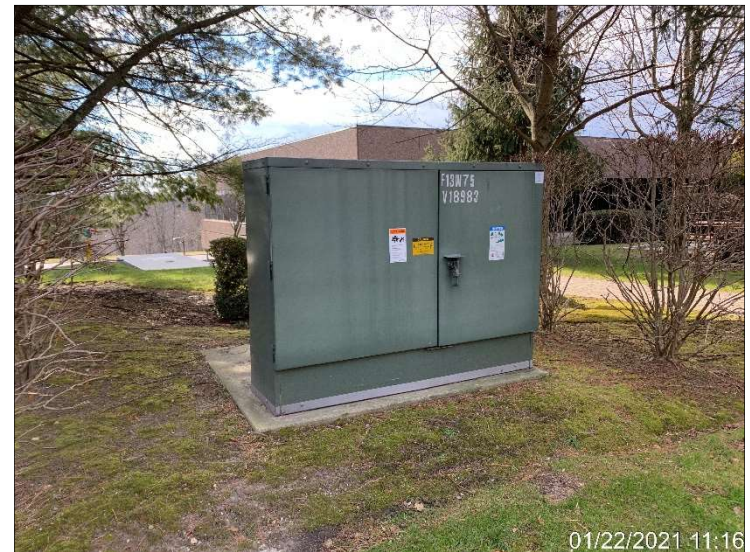
Photograph 24. Pad-mounted transformer in a landscaped area behind Building 2.
