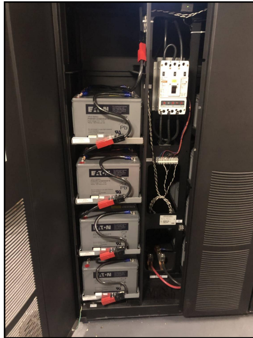
7 : Lead batteries for backup power
