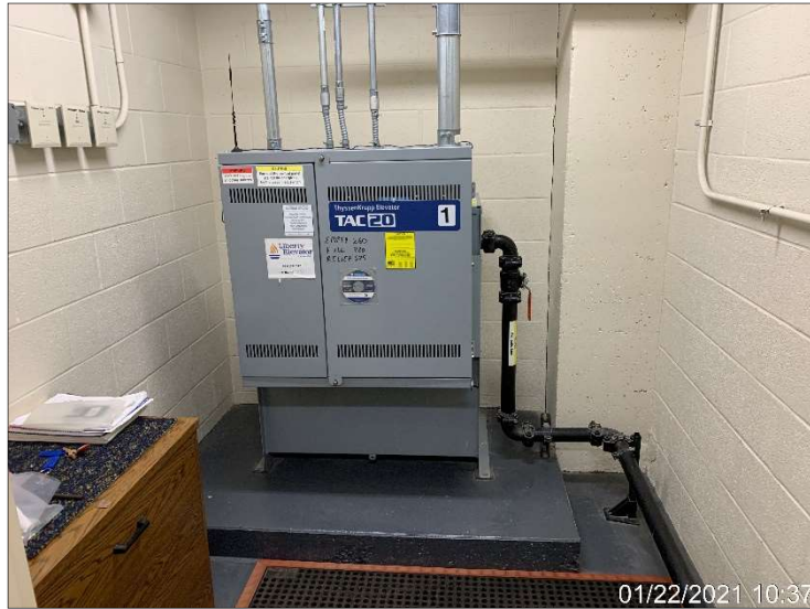
Photograph 21. Hydraulic equipment in the elevator machine room in the cellar of Building 2.
