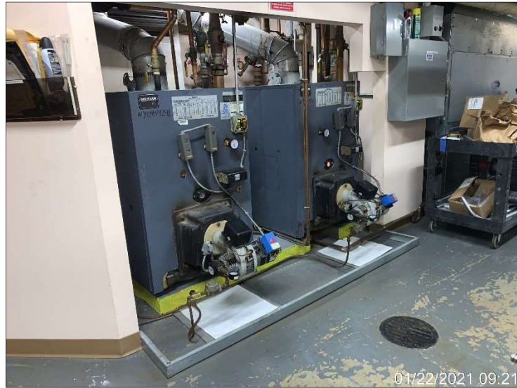
Photograph 5. Two No. 2 fuel oil-fired boilers in the boiler room on the 1 st floor of Building 1.
