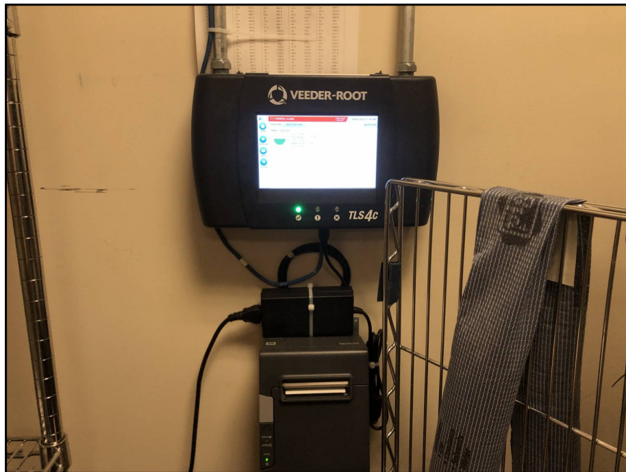
18 : Veeder-Root UST leak detection monitoring system for Building No. 1
