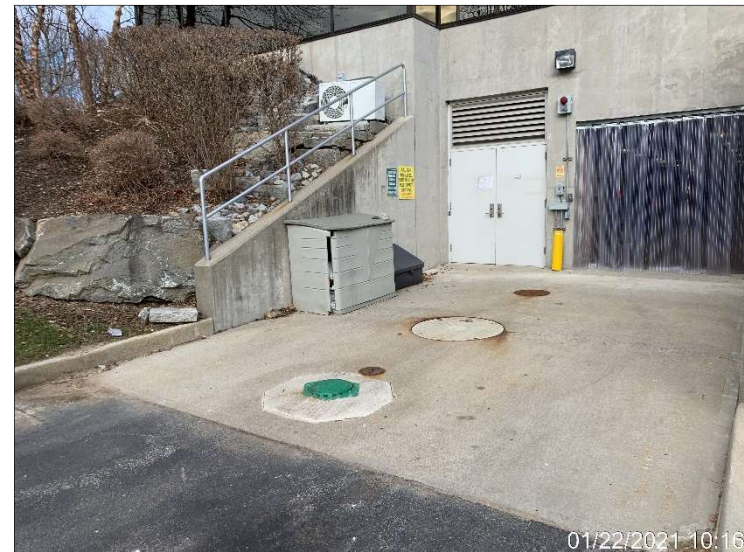
01/22/2021 10:16 Photograph 20. 2,500-gallon No. 2 fuel oil tank (Tank No. 002) serving Building 2, located outside the southeastern portion of the building.
