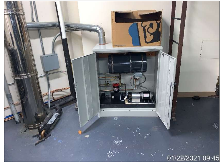
Photograph 6. Fuel oil transfer pump for the boiler system, located in a mechanical room on the 2 nd floor of Building 1.
