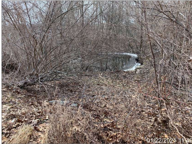
Photograph 33. One of two stormwater detention basins located south of the office complex.
