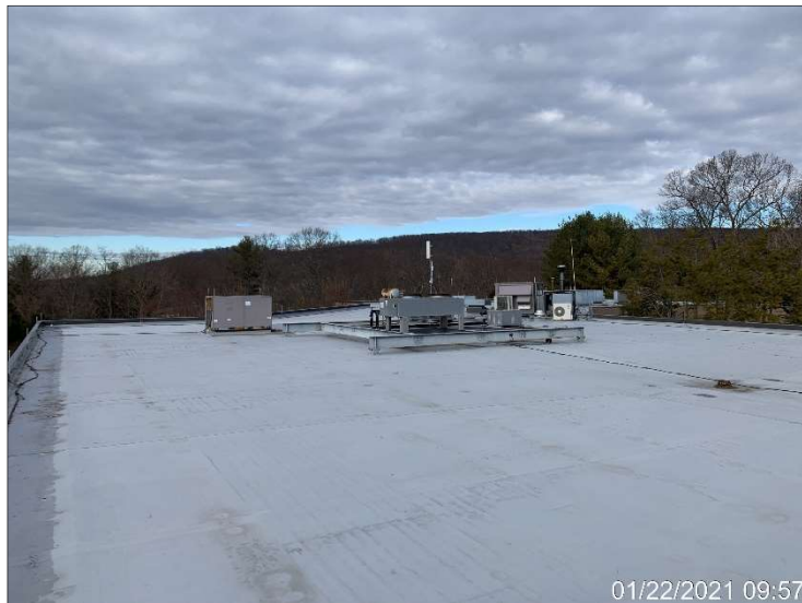
Photograph 11. HVAC equipment on the roof of Building 1.
