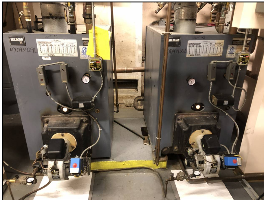
10 : Oil-fired boilers in Building No. 1
