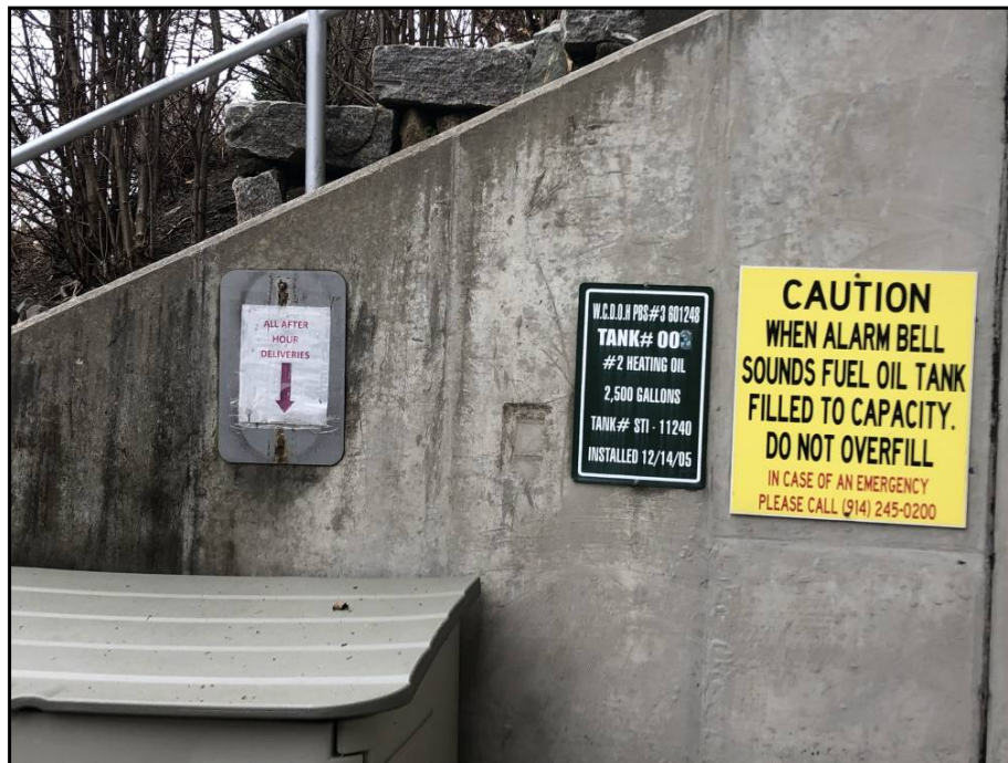
15 : 2,500-gallon fuel oil UST for Building No. 2
