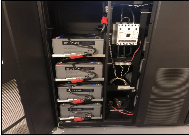
Lead batteries for backup power
