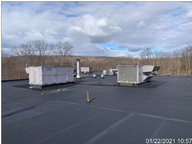
Photograph 23. HVAC equipment on the roof of Building 2.
