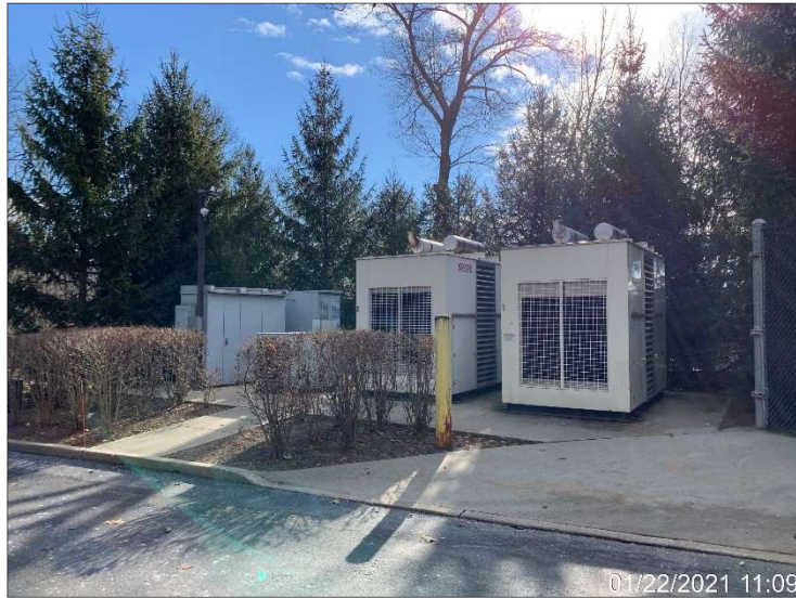
Photograph 29. Two emergency generators with self-contained 50-gallon No. 2 fuel oil ASTs (Tank Nos. 004 and 005), located east of the office complex.
