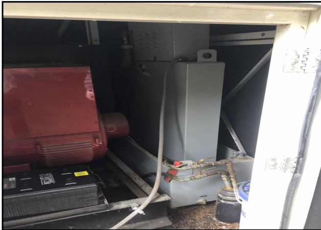
View of 50-gallon AST associated with each emergency generator
