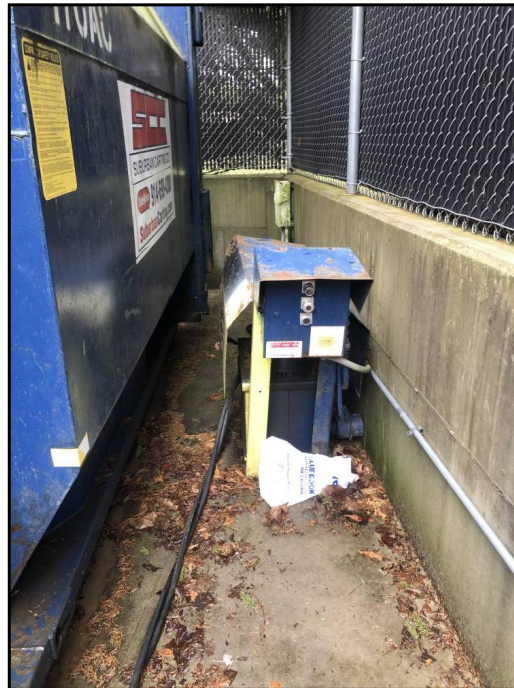
22 : Hydraulic oil storage unit associated with trash compactor
