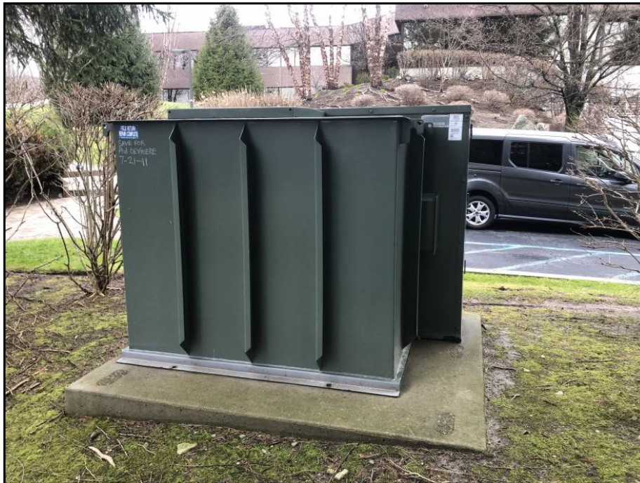
20 : Pad-mounted transformer for Building No. 2
