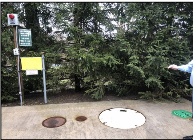
1,000-gallon Fuel Oil UST for emergency generators
