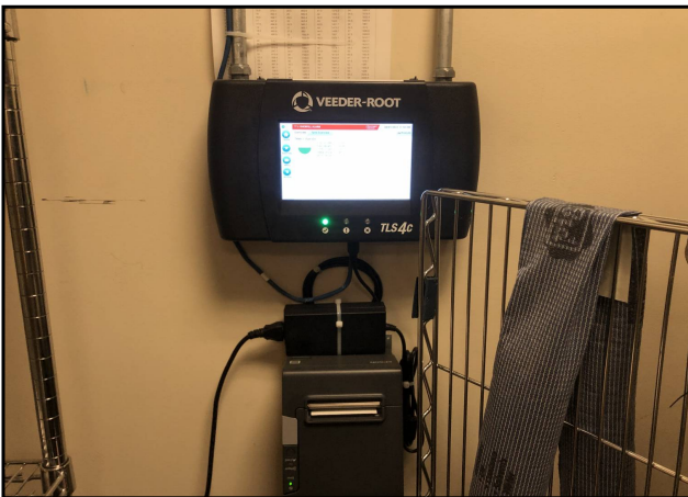
Veeder-Root UST leak detection system for Building No. 1
