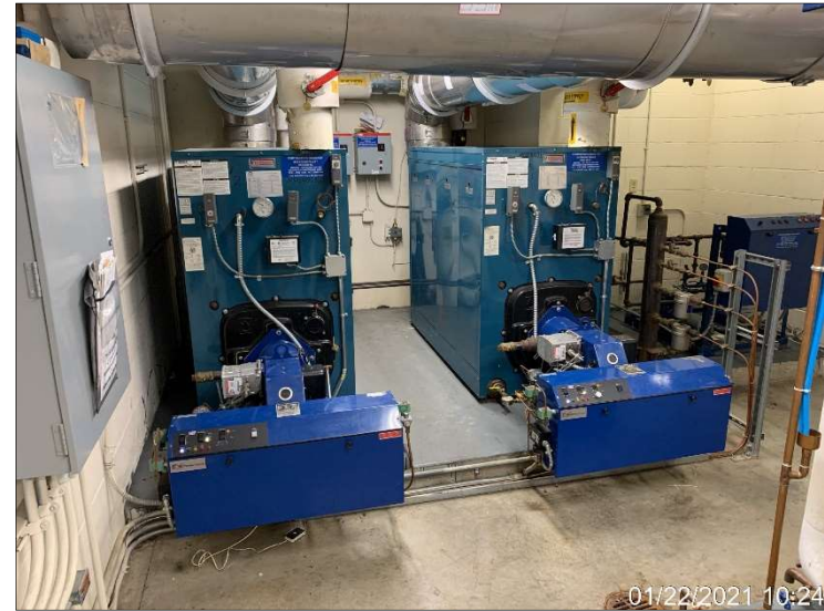
01/22/2021 10:24 Photograph 18. Two No. 2 fuel oil-fired boilers in the boiler room in the cellar of Building 2.
