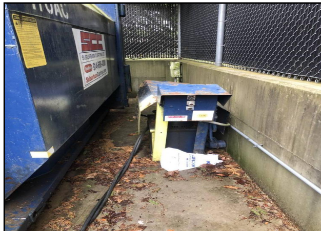
Hydraulic oil storage unit associated with trash compactor
