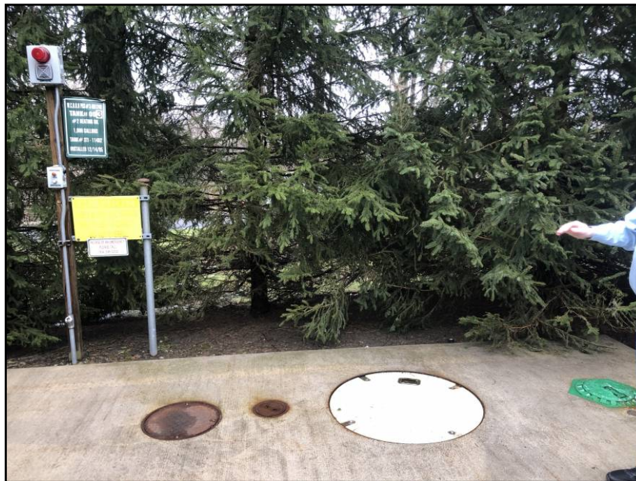
16 : 1,000-gallon fuel oil UST for emergency generators
