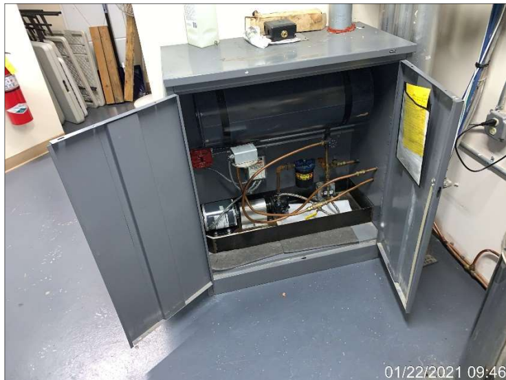
Photograph 7. Backup fuel oil transfer pump for the boiler system, located in a mechanical room on the 2 nd floor of Building 1.
