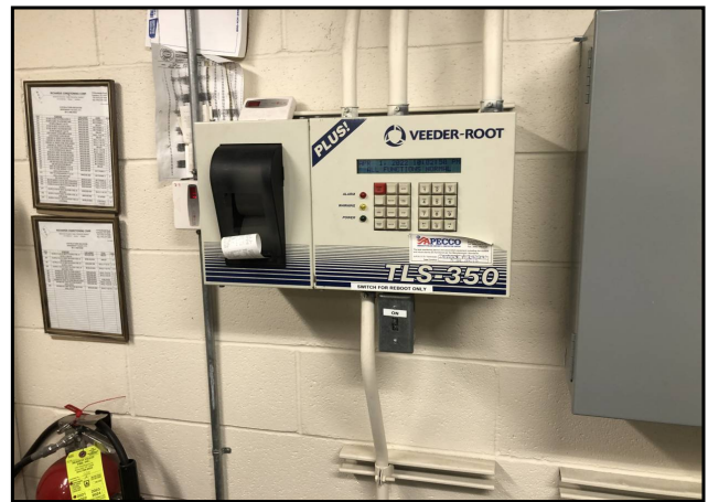
Veeder-Root UST leak detection system in Building 2
