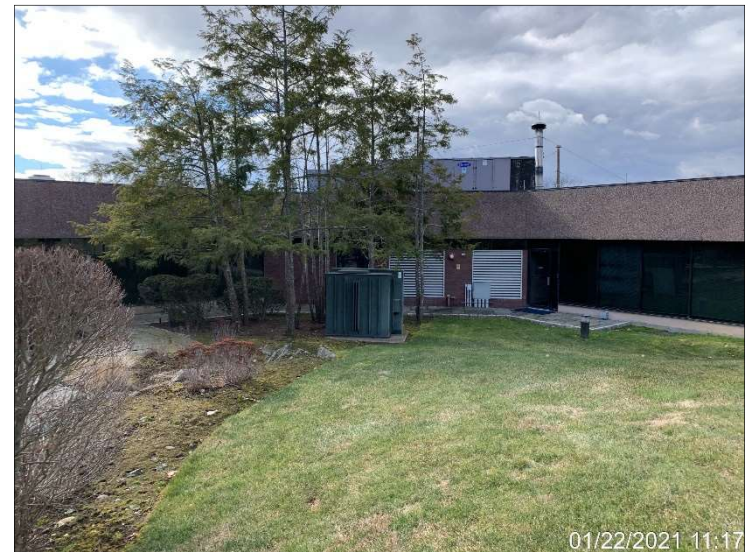
Photograph 12. Pad-mounted transformer in a landscaped area behind Building 1.
