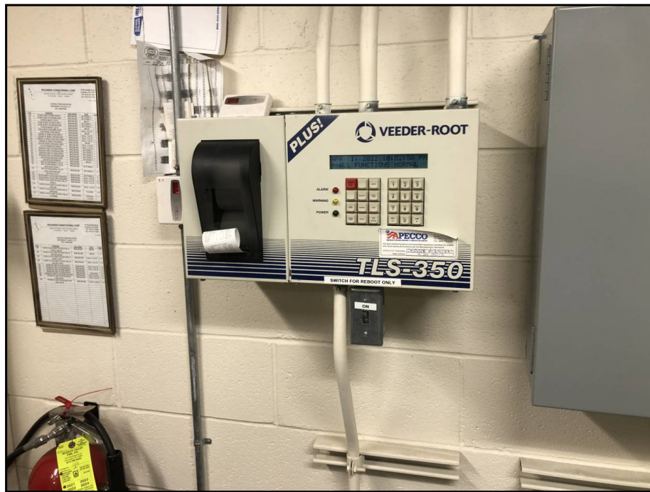
17 : Veeder-Root UST leak detection monitoring system in Building No. 2
