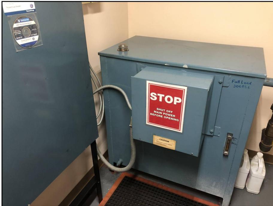
12 : Hydraulic elevator equipment in Building No. 2
