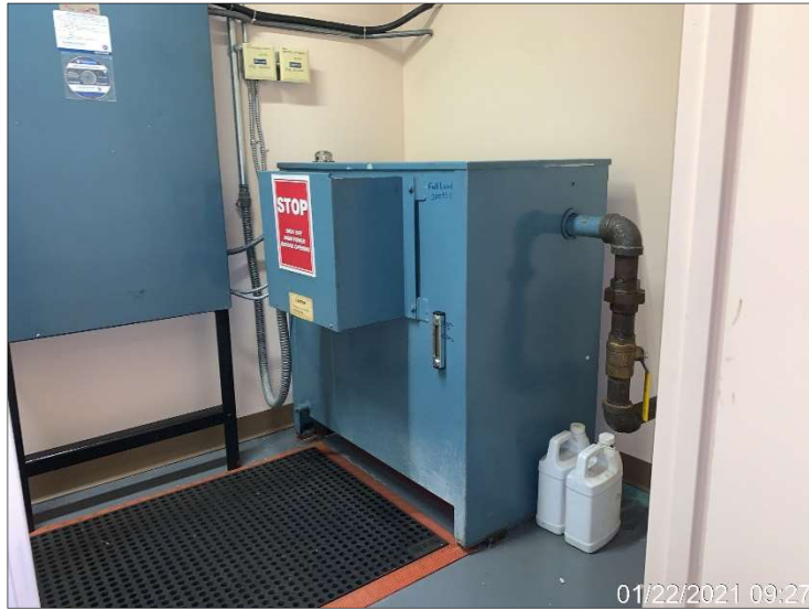
Photograph 9. Hydraulic equipment in the elevator machine room on the 1 st floor of Building 1.
