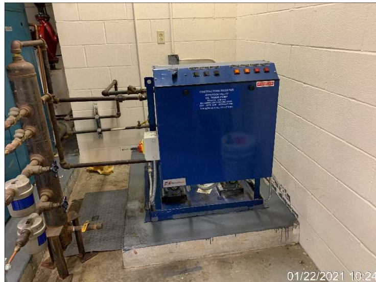
01/22/2021 10:24 Photograph 19. Fuel oil transfer pumps for the boiler system, located adjacent to the boilers.
