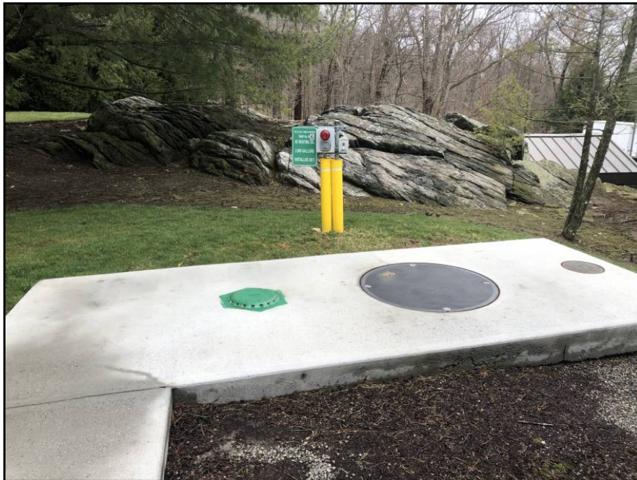
14 : 2,000-gallon fuel oil UST for Building No. 1
