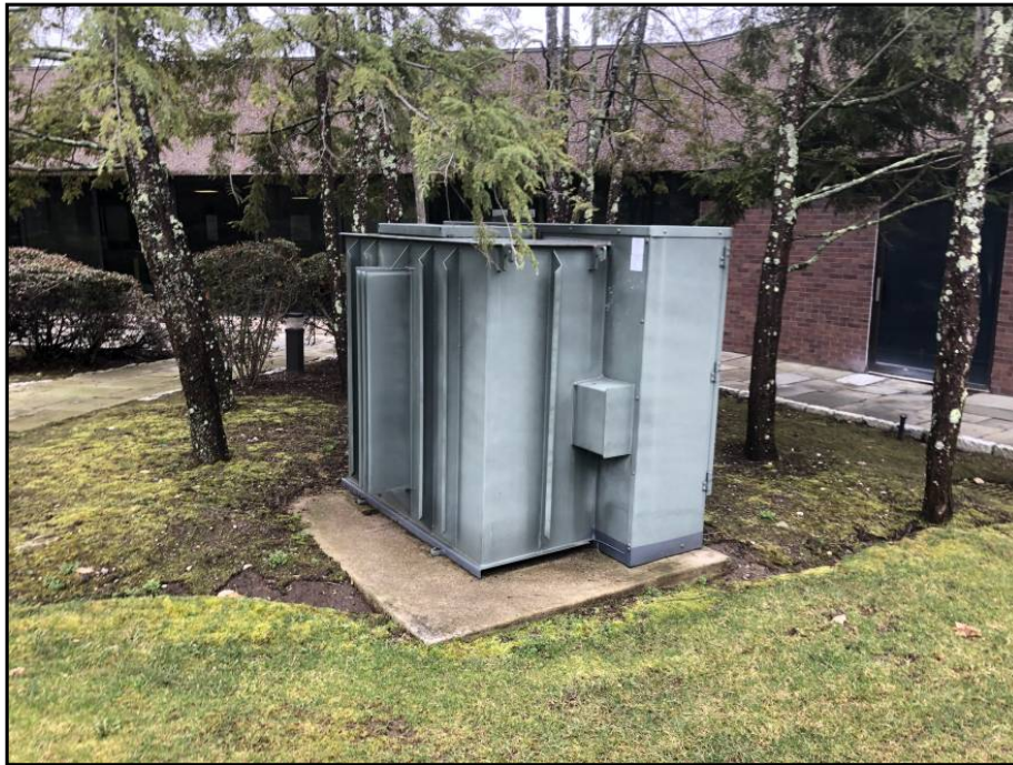
19 : Pad-mounted transformer for Building No. 1
