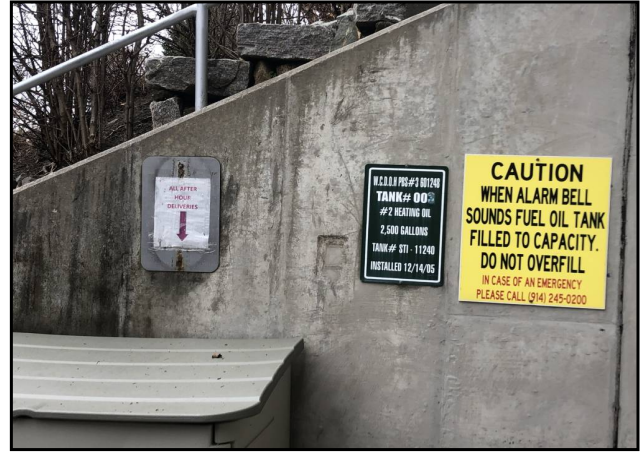
2,500-gallon UST for Building No. 2
