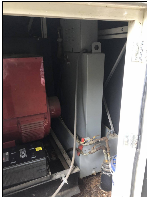
24 : 50-gallon AST within each emergency generator
