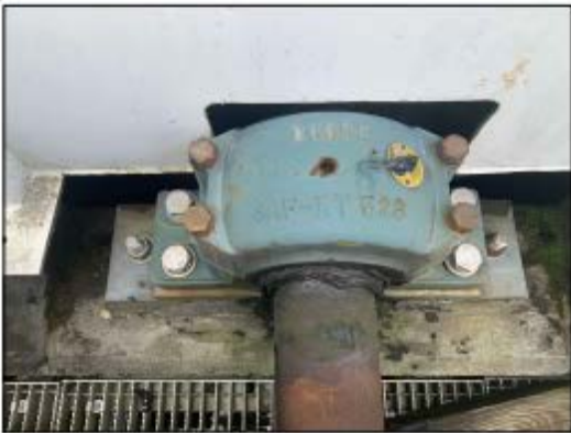
TYPICAL IDLER BEARING
