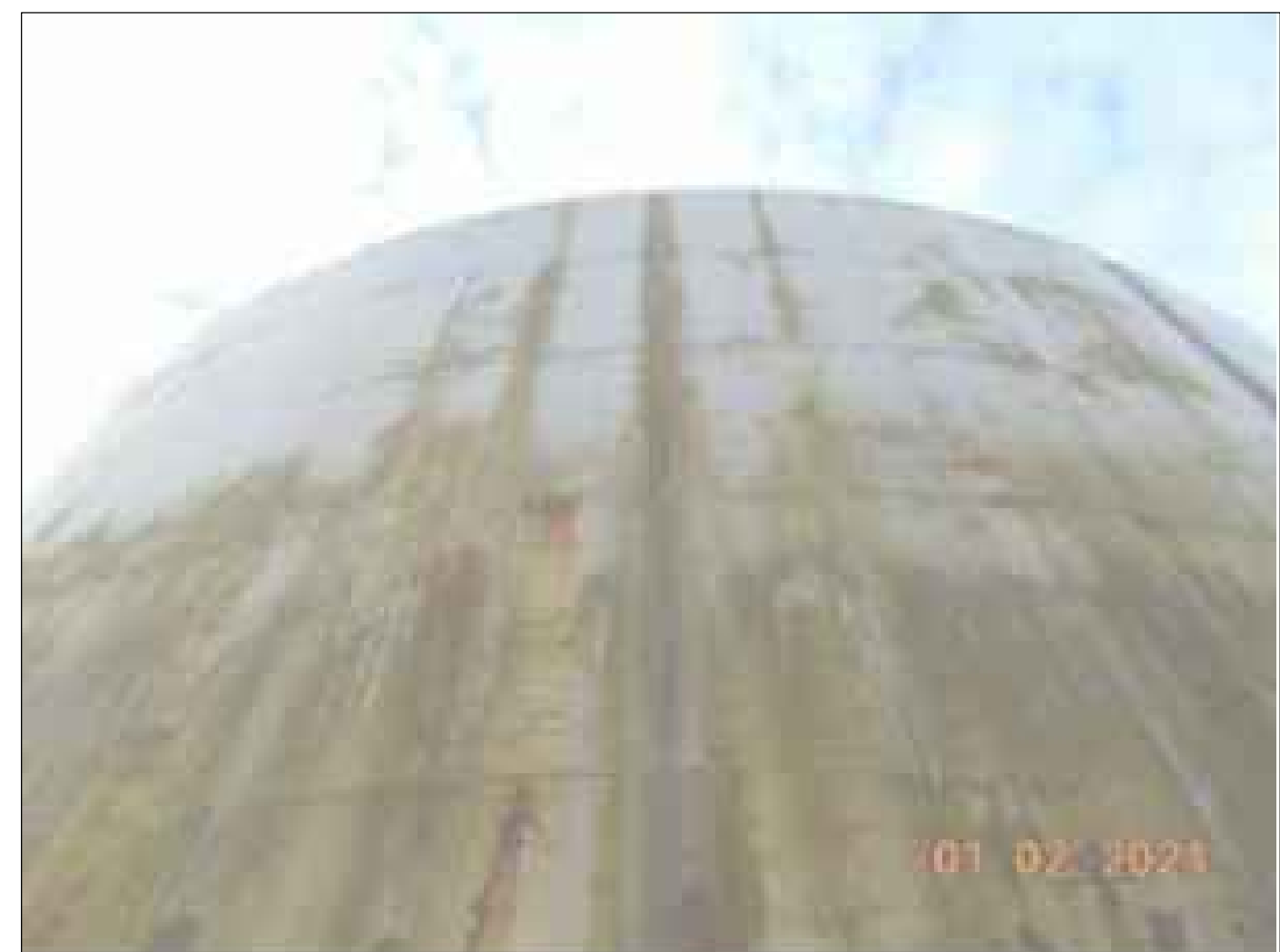
7 BIOLOGICAL STAINING AND CORROSION ON THE SHELL NOT TO SCALE
