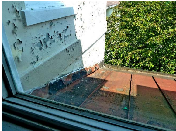
East wall of 1924 Addition: peeling paint and visible staining on concrete walls; original Porch roof and flashing with repairs
