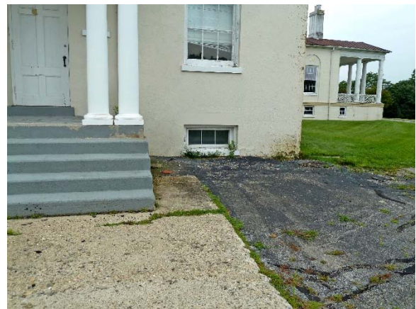
Chapel, east elevation: peeling paint along northeast corner of building & concrete stair; macadam driveway with repairs
