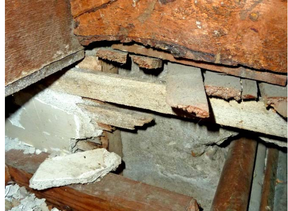
Kitchenette: floor probe exposes plaster walls above a dropped ceiling, and concrete wall penetration
