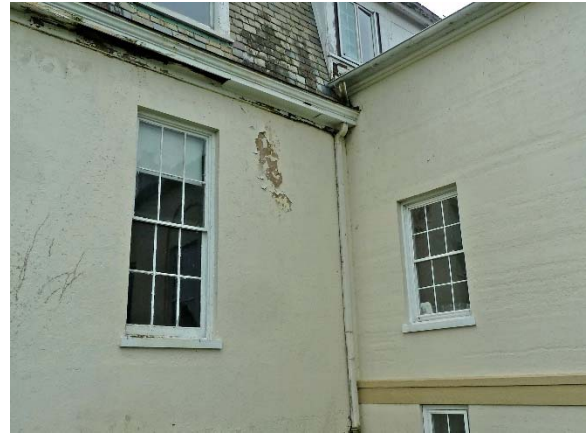
Chapel, north elevation: roof soffit very deteriorated and open; peeling paint on wall; downspout at corner with pavilion
