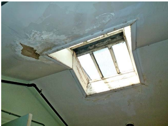
Records room at East Pavilion stair landing: deteriorated ceiling plaster, peeling paint, replacement glazing
