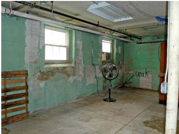
East wall of basement below South Pavilion: deteriorated wall finish; peeling paint, leak kindly identified
