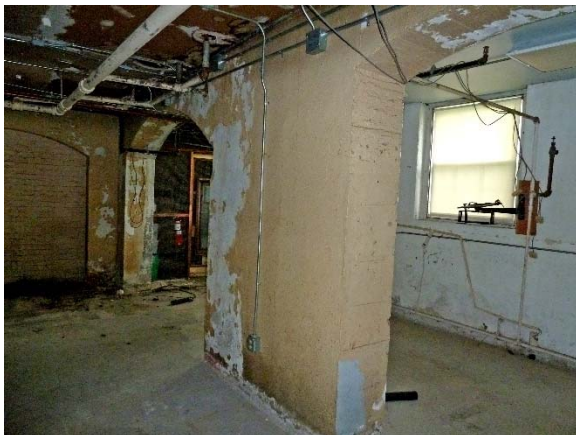
Structural arches outside elevator mechanical space (south rooms); peeling paint; deteriorated & stained ceiling boards
