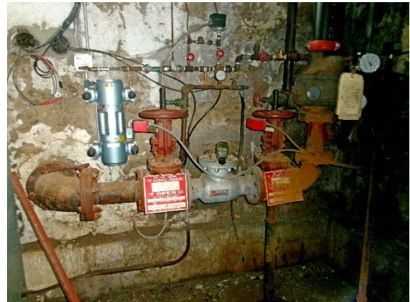
Basement mechanical room: controls for sprinkler system
