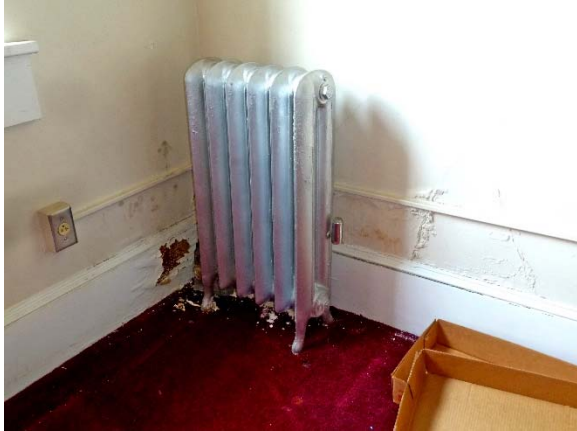
Peeling & bubbling wall and baseboard finishes around steam radiator suggests ineffective or failing controls
