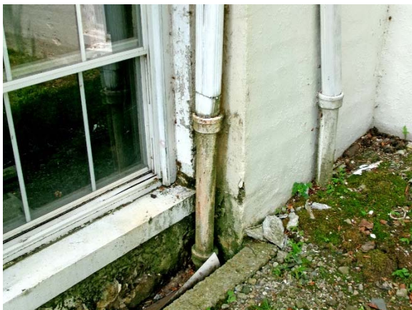
Drainage trench outside basement windows at western end of façade; significant mildew/moss; water infiltration to interior
