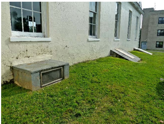
Chapel, south elevation: peeling paint and repairs at lower walls; access point to basement level
