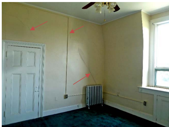
North bedroom near joint with East Portico: severe cracks along entire wall (typical both sides of room)
