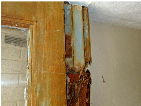
Exterior basement door, at West Elevation: steel frame severely rusted & disconnected with bird nest inside
