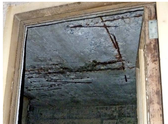
Underside of West first floor entry portico: concrete slab with multiple rebar visible & rusty near the deteriorated surface
