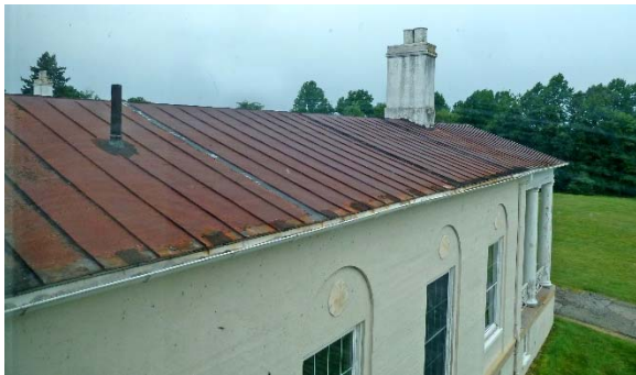
East Pavilion roof (likely original standing seam, 1924); at end of service life with numerous repairs/rust; gutter drooping
