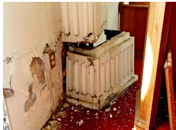
Chapel, south wall by sanctuary: sheet metal pilaster/tie cover disconnected; peeling paint on exterior wall and cover
