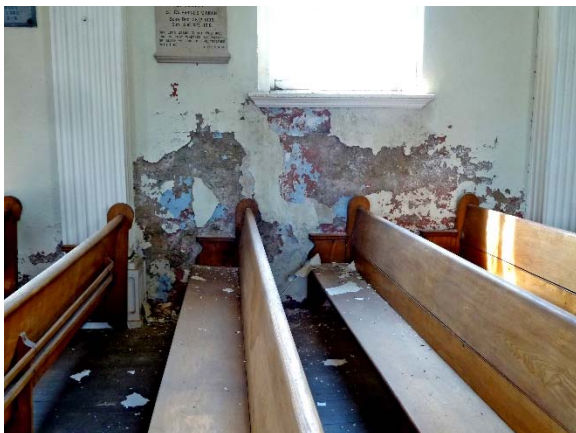
Chapel, south wall: severely deteriorated finishes below window sills, allowing view of previous paint layers & bare concrete
