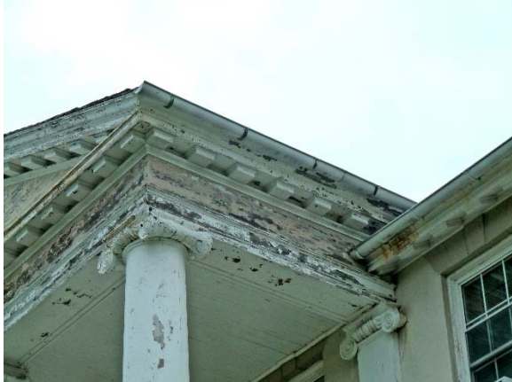
Details of portico: flaking paint at entire wood pediment, entablature & columns; staining below main façade gutter
