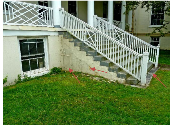
North porch stairs: visible structural cracks on side wall(s); displaced & rotated lowest two stairs/treads; peeling paint
