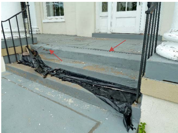
Portico floor: deteriorated/spalling concrete stair edge, uneven pavers, peeling paint (floor & ceiling above)
