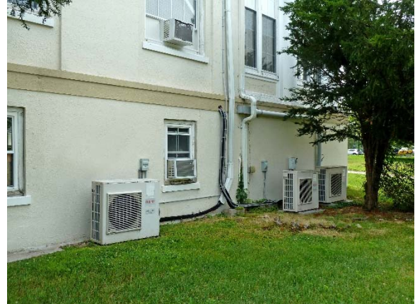
In-window air conditioning units; multiple split system condensing units with conduit overlapped by downspout
