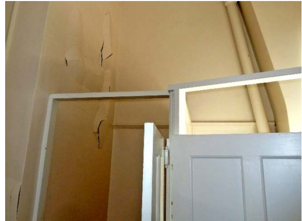
Bathroom at western end of hall: painted finishes bubbling, settling, and falling off at partition wall to linen closet
