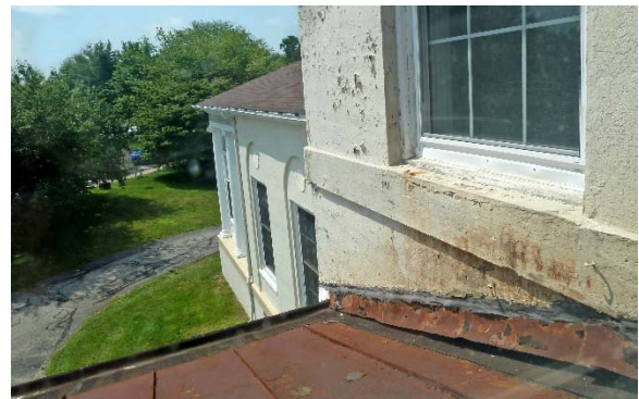
East wall of 1924 Addition: peeling paint and visible staining on concrete walls; original porch roof and flashing with repairs
