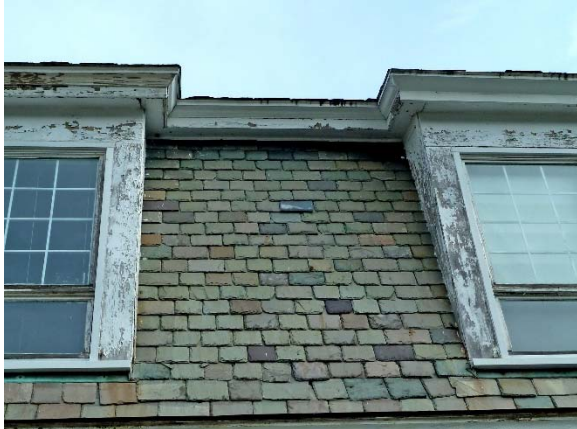
Chapel, south elevation: Slate gambrel roof in fair condition with some slates slipping or displaced; peeling dormer trim
