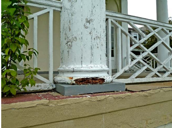
East Pavilion: extremely deteriorated torus of column along north façade; porch floor covering peeling away
