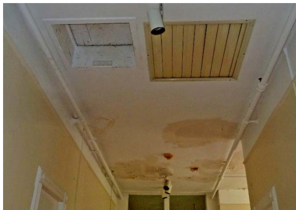
Central Addition (1924), hall near central stair: water-stained ceiling; access panel to attic and louvers to whole-building fan
